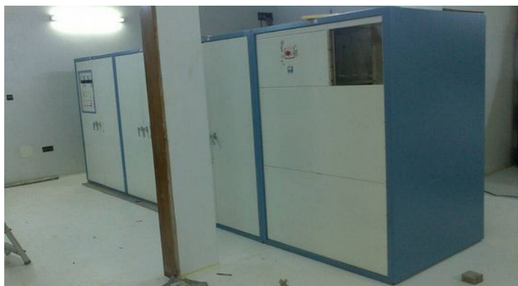
Transmitter in place awaiting equipment in containers
