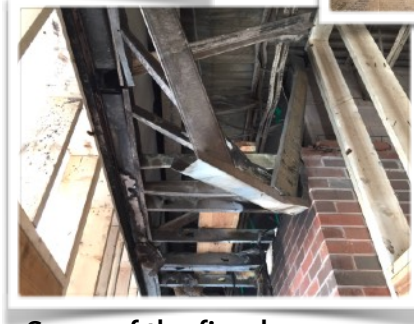
Some of the fire damage.
