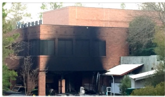
Southwest Corner where the fire started.
