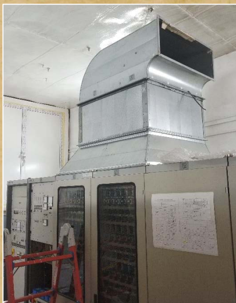
The above left frame was one of many fabricated to fit into the overall transmitter cooling system (right), to provide proper ventilation for the transmitter.
